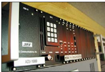
Communications and interoperability are the key to any mobile command post.
