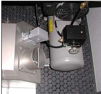
Air filtration system
